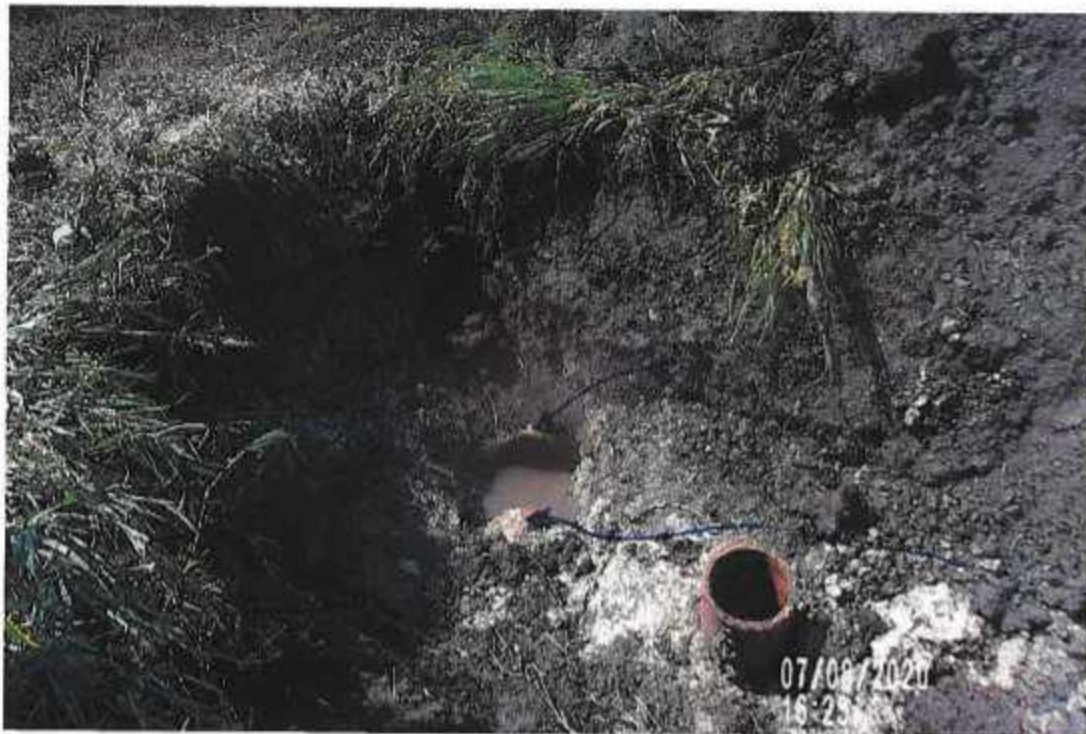
PICTURE# 4068 IS LOOKING NW SHOWING TILE FLOWING IN SOUTH DITCH OF CO. HWY D41
