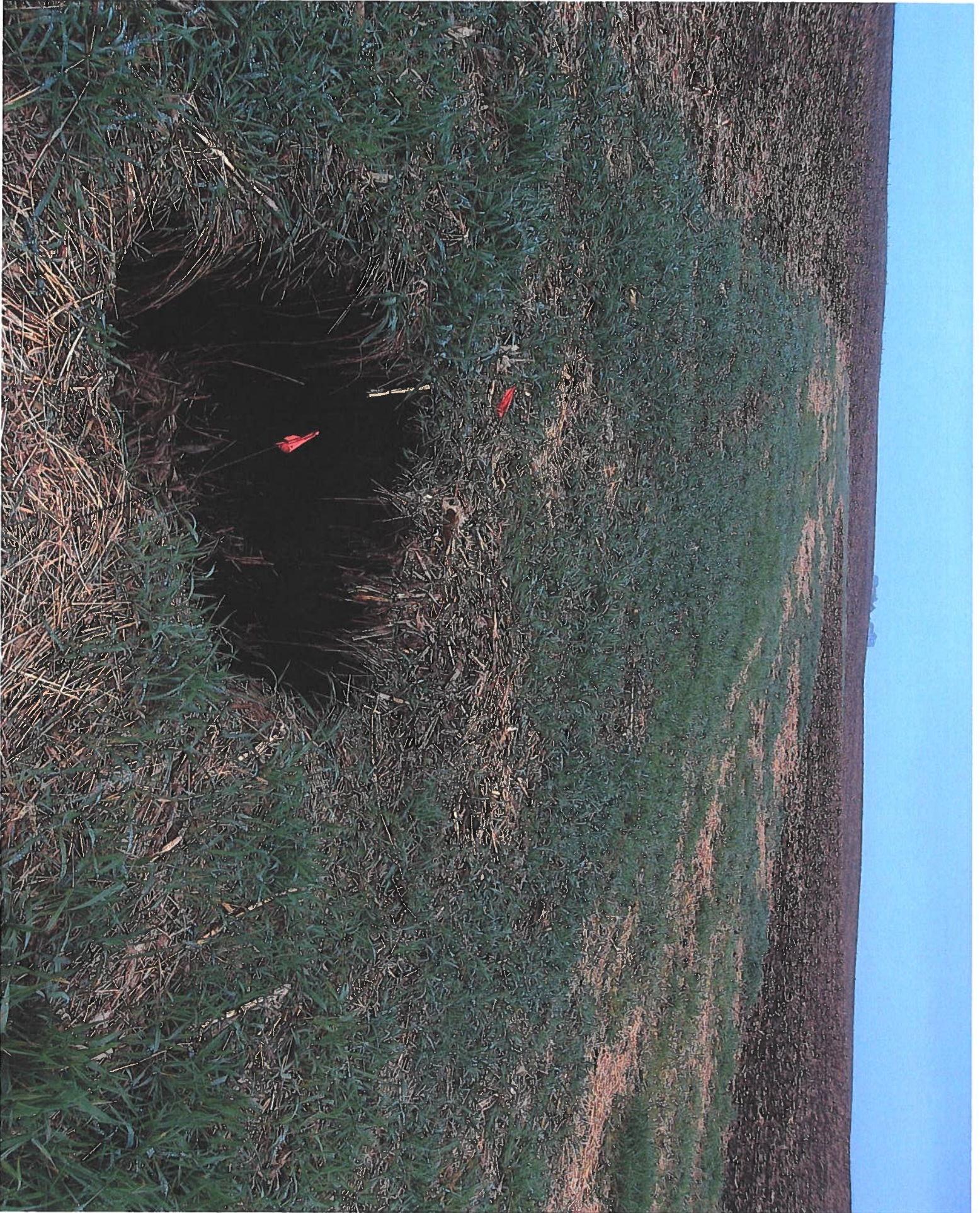
NORTHERN MOST Blow-out, COLLAPSED TILE 15" \phi ±
