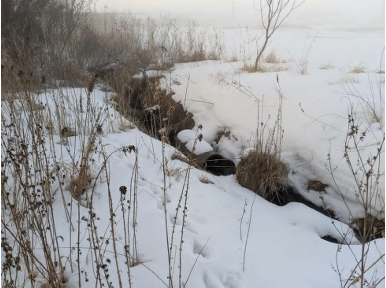
Figure 1: 1922 Main completely exposed and broken above outlet.
