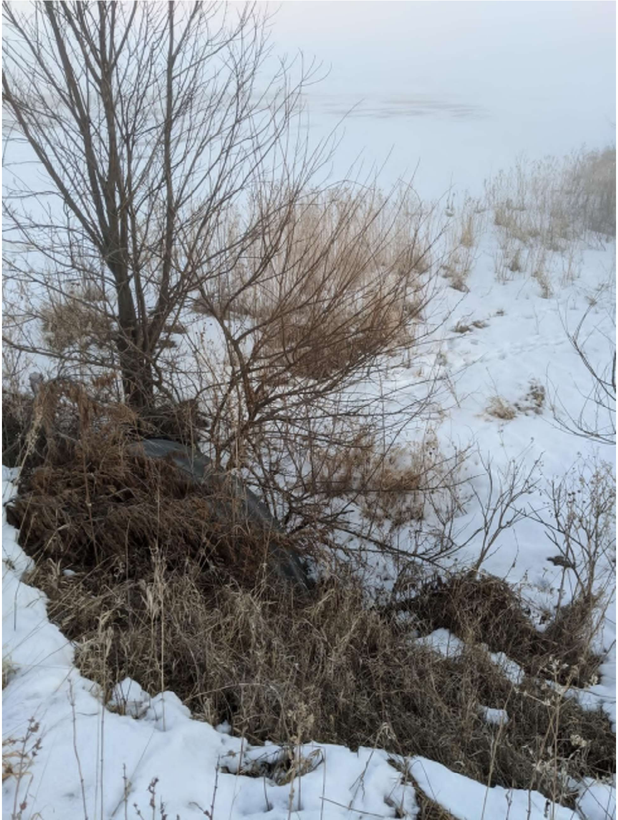
Figure 5: Trees and woody brush over lower 100 feet of 1922 Main tile.
