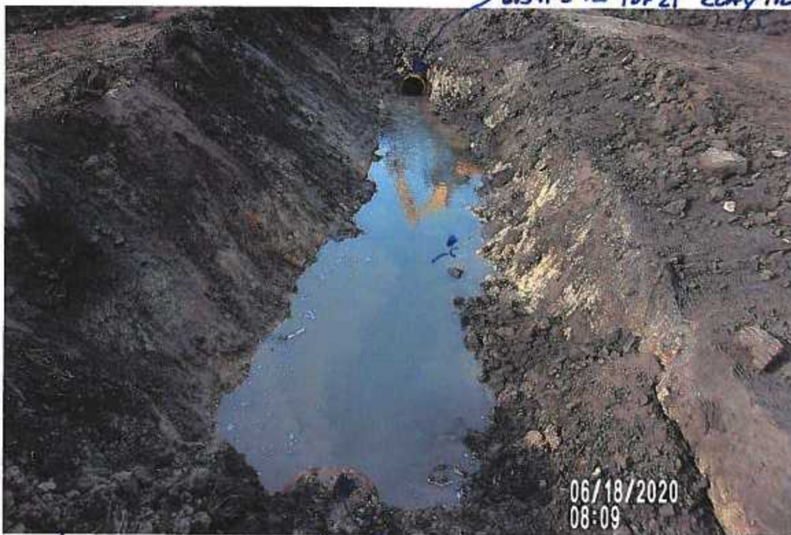
(TEMPORARY REPAIR) PICTURE# 3819 GPS# 394 TILE TOP 21" CLAY (1.72' TOP TO FL) IS LOOKING SOUTH UPSTREAM 5.4'± DEEP WITH MUCK CLEANED OUT OF BOTTOM OF TRENCH & READY TO INSTALL 24" HOPE DW NONPERF TILE. BOTTOM IS SOFT IN AREAS AND WILL USE SOME ROCK TO FIRM UP ON INSTALLATION
