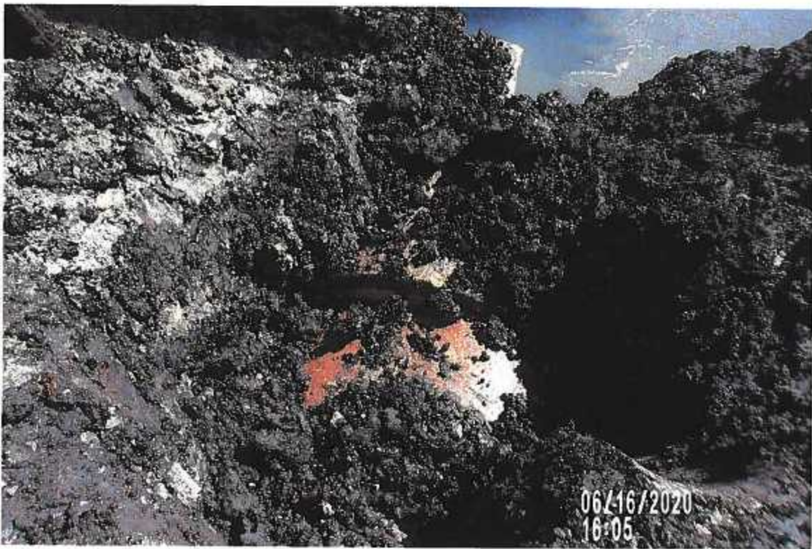
PICTURE #3789 IS LOOKING SOUTH SHOWING TILE CAVING DOWN 5.0' DOWN STREAM FROM GPS#393.
