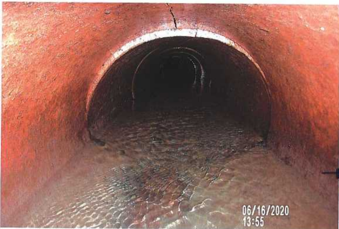
PICTURE # 3779 IS LOOKING SW UPSTREAM FROM GPS#392. INSIDE - 21" CLAY TILE WITH SMOOTH CRACKS @ 6 & 12 O'CLOCK, TILE IS CRACKED, SLIGHTLY SQUATTED, BUT DOES NOT APPEAR TO BE LEAVING DOWN.
