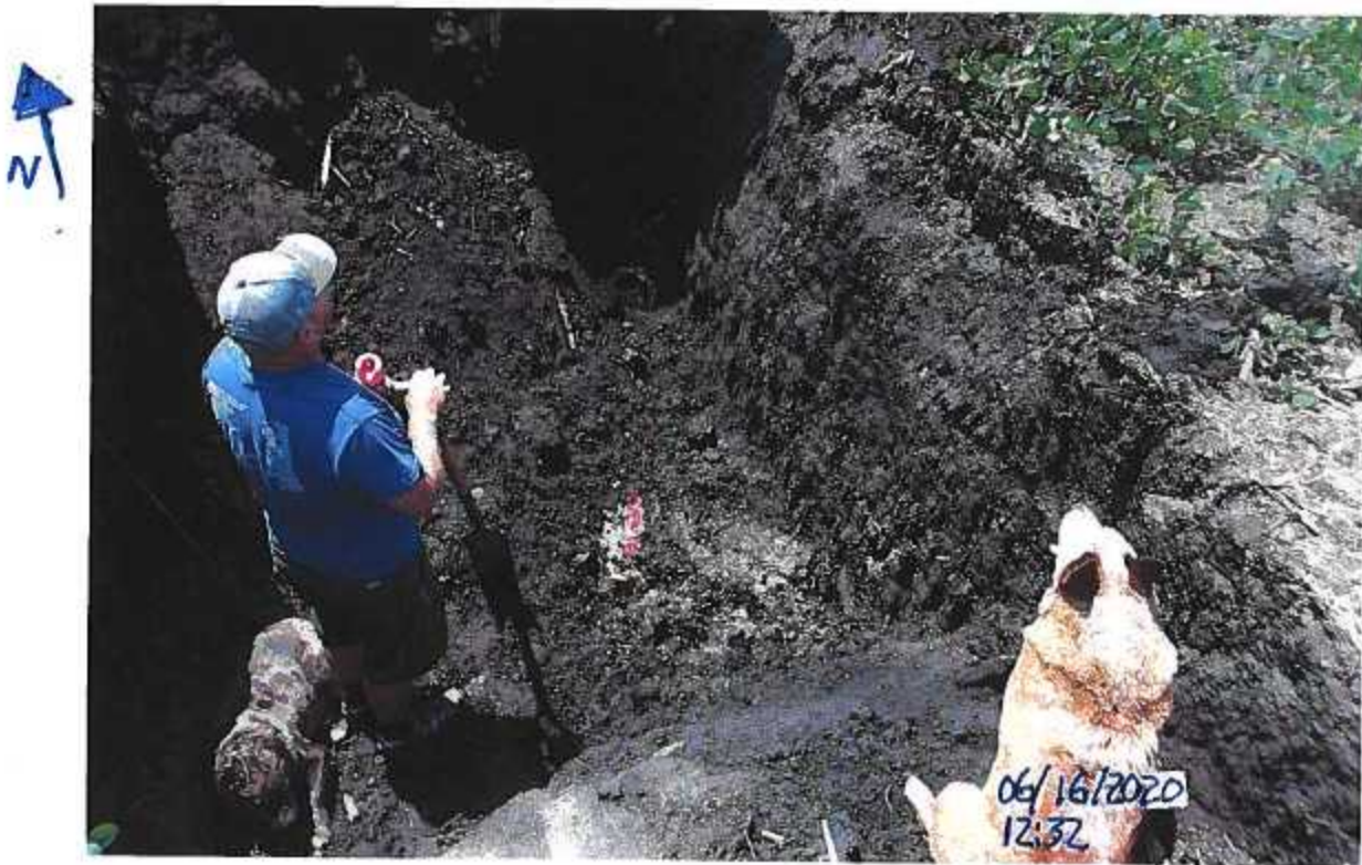
PICTURE # 3778 IS LOOKING NE SHOWING TILE EXPOSED WHERE SECTION OF TILE IS BROKEN & COLLAPSING NEAR BLOWOUT HOLE,
