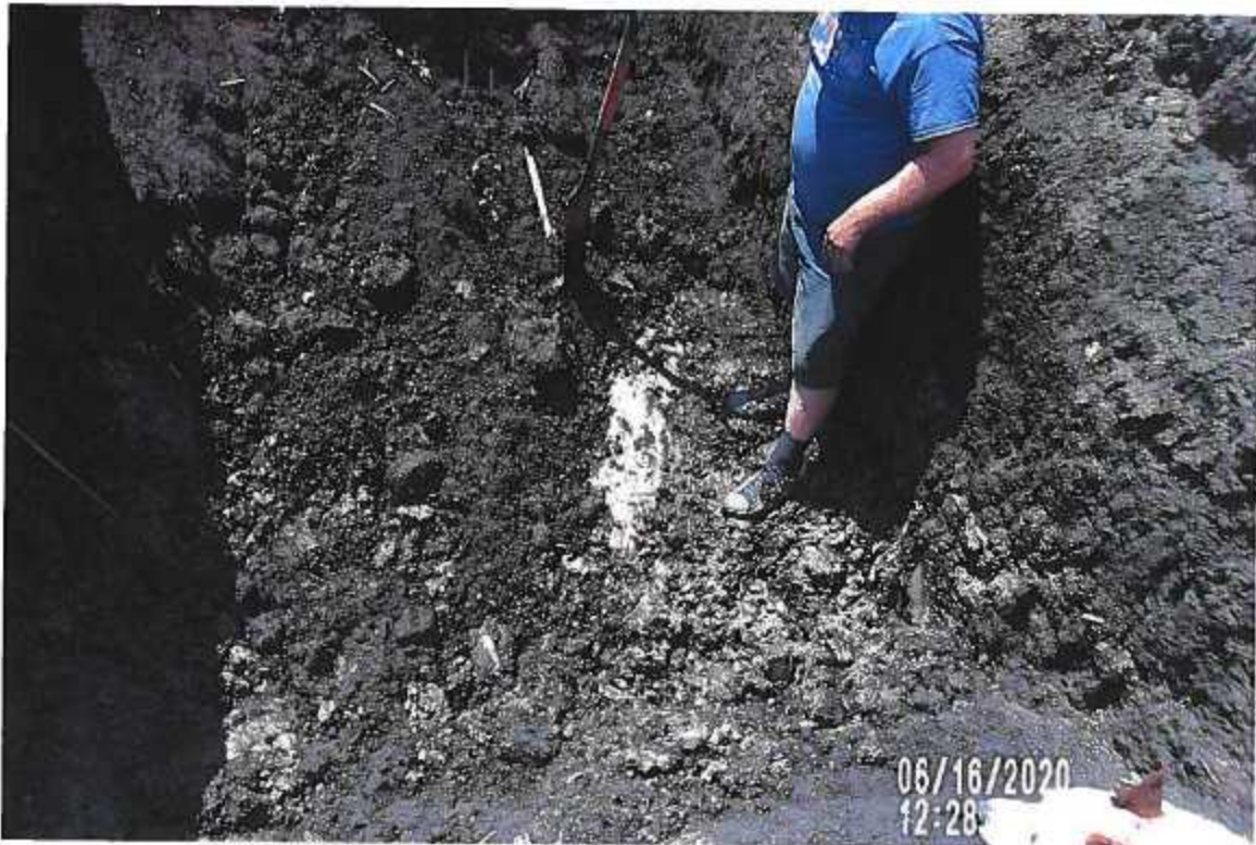
PICTURE #3776 IS LOOKING SW SHOWING EXISTING CLAY TILE EXPOSED NEAR TILE BLOWOUT WITH NO VISIBLE ISSUES YET (JOINT IS TIGHT)
