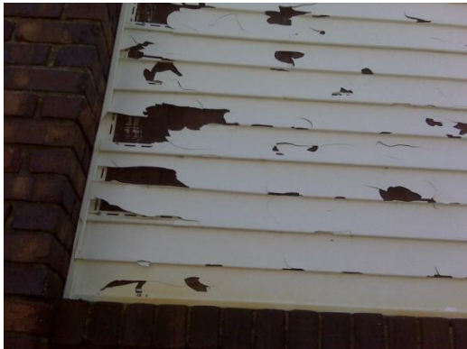
Hail damage to vinyl siding, August 2009, Eldora, Iowa.
